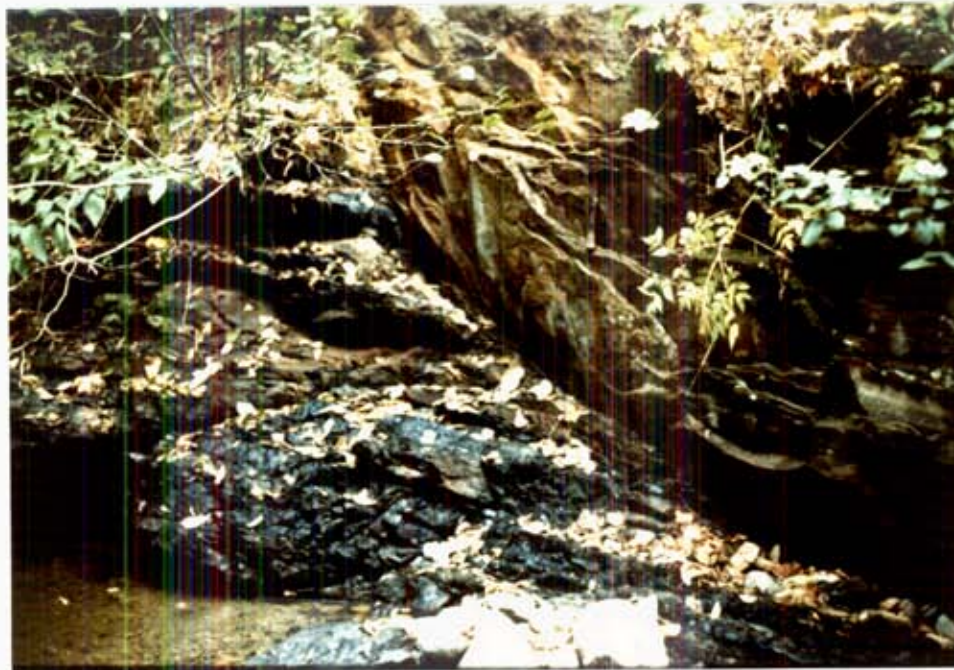
PLATE I: Major normal fault feature on Dove Creek approximately 1.6 km west of the Anderson East Licence Area. Note coal seam in faulted contact with the sandstones of the down-faulted block. Photo looking north.
