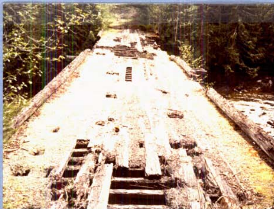
Plate 2: Outcrop 2. Note condition of bridge. Impassable for drilling rigs.
