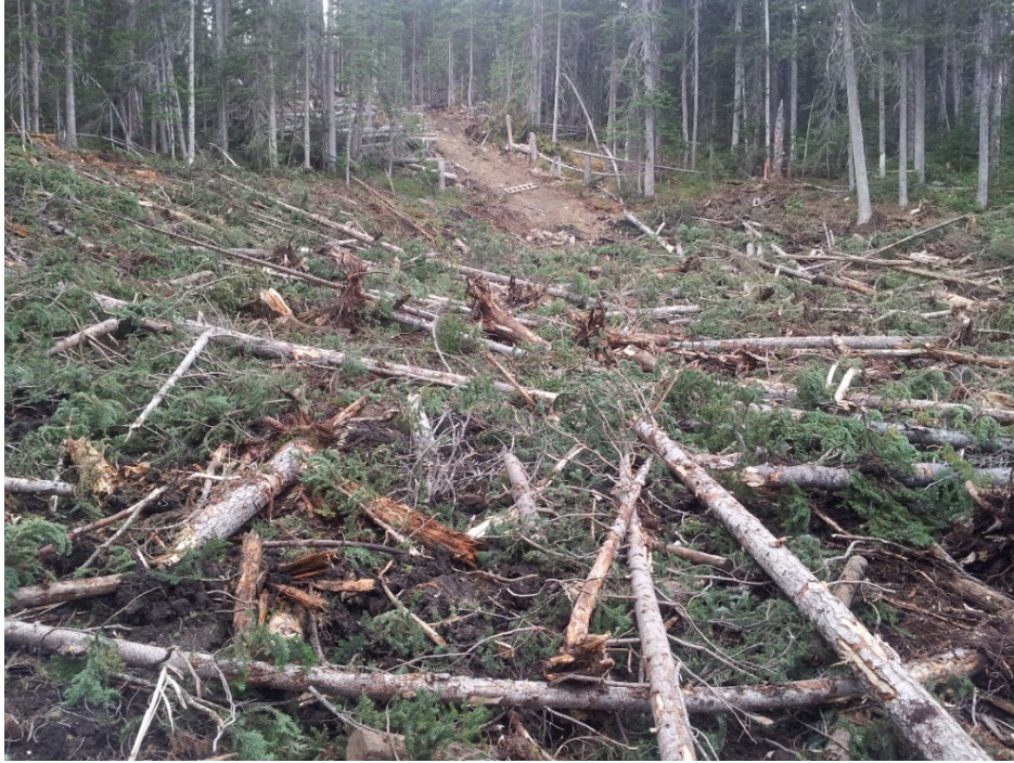
Figure 13: Photograph of trench site after organic material has been spread over the entire trench site.
