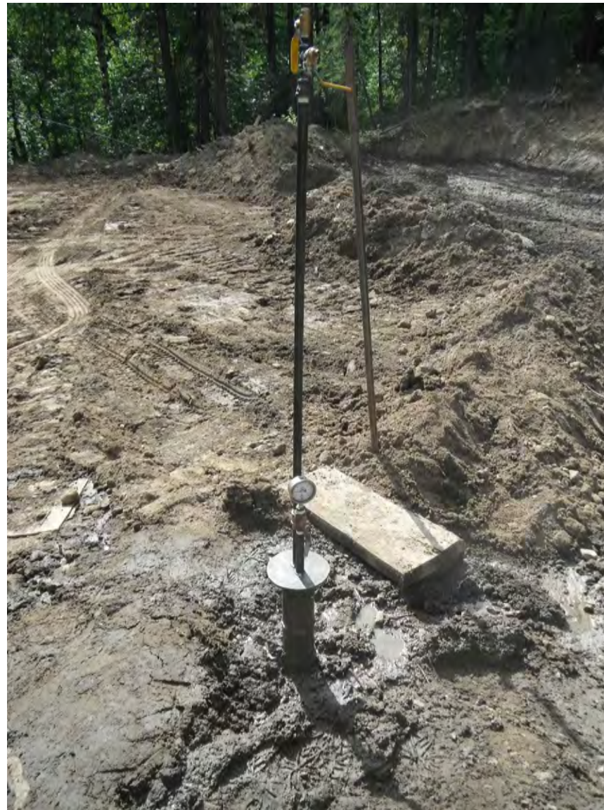
Photo 2: Photo shows two 19 mm diameter steel pipes extending above grade from the threaded HQ top cap. The shorter of the 19 mm diameter steel pipes is capped with a pressure gauge and the taller of the 19 mm diameter steel pipes is capped with a pressure release valve such that methane gas can escape from the system.
