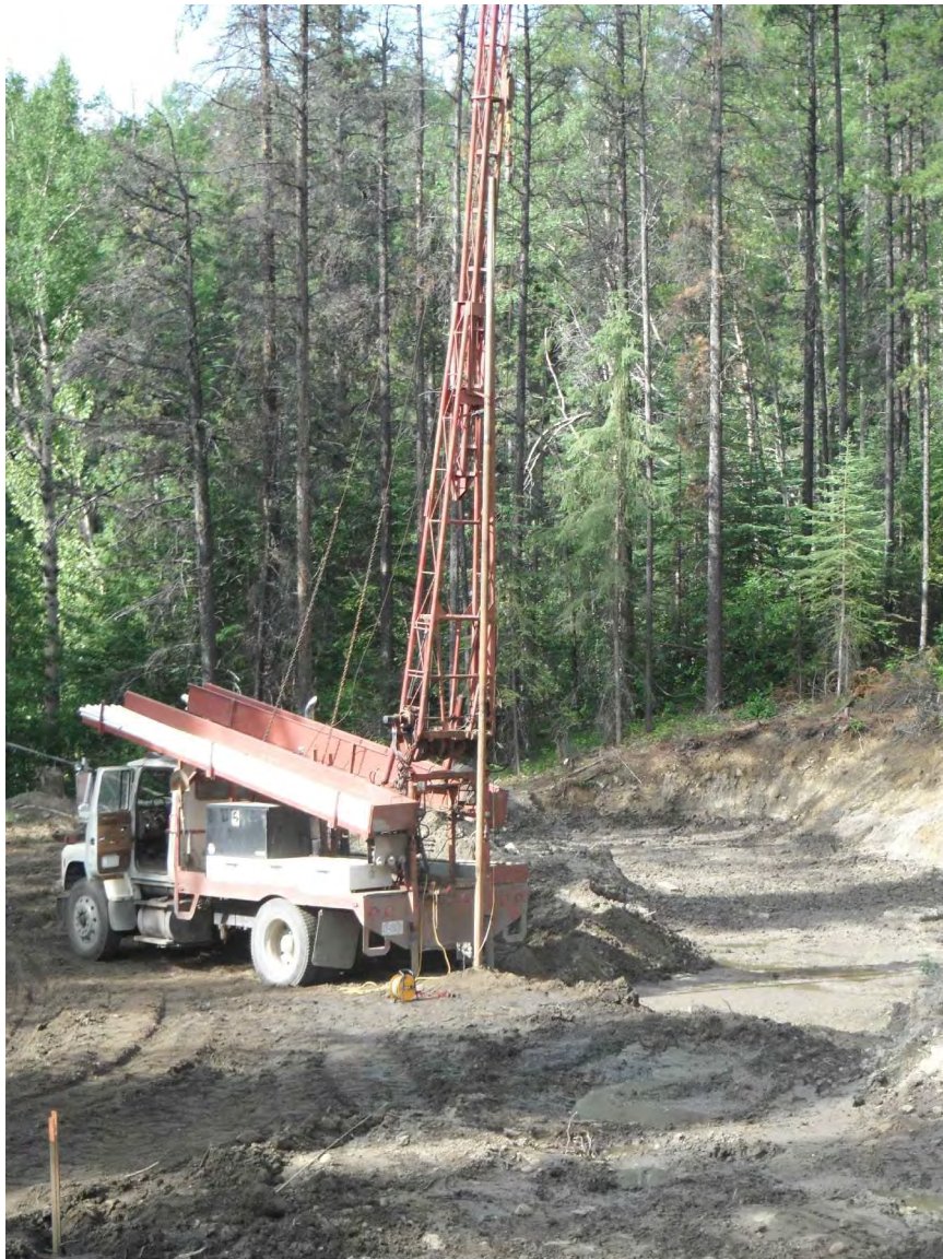
Photo 1: View toward the south southeast from Borehole H16W. The drill rig in the centre of the photo is supporting 9.1 m of HQ drill rod (above-grade) threaded into the top of Observation Well H16. Groundwater is flowing over the top of the extended drill rod.
