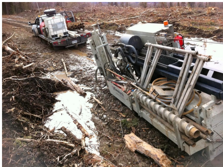
Plate 1. Poor road conditions into the work site; stuck drill rig and the truck.
