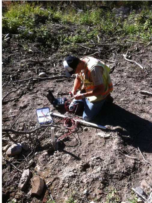
Plate 3. Monitoring vibrating wire piezometer MW-H12.
