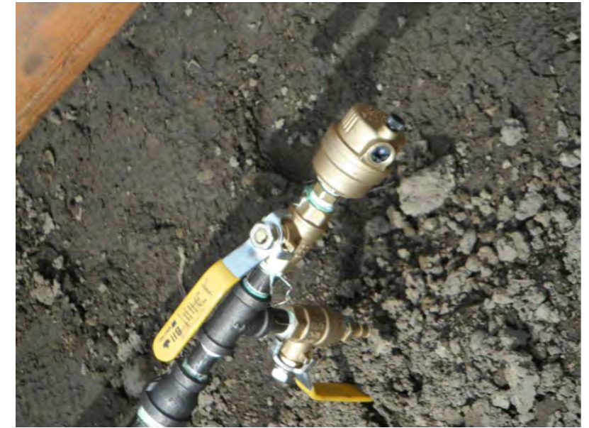
Photo 3: Close-up photograph showing the detail of the pressure release valve threaded into the top of the longer 19 mm diameter pipe. The yellow handles are ball valves to release water from the system when the groundwater head rises too high in the system.
