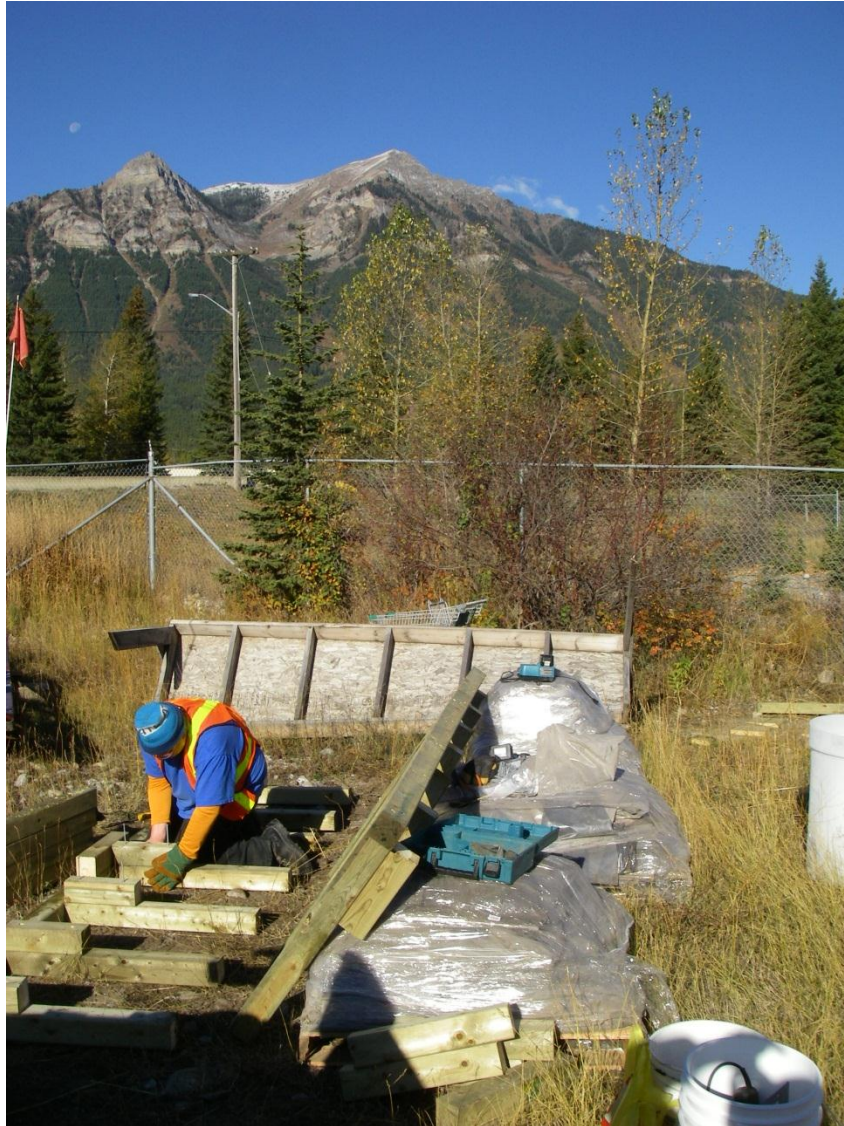
Figure 4: Construction of Support Structure, with Sample Materials (Wrapped on Pallets) and Field Cells (Far Right)
