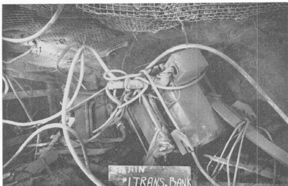
Plate XIIA. Balmer North mine. Transformer bank on No. 3 main showing force of the explosion. (Courtesy of Crows Nest Industries Limited.)
