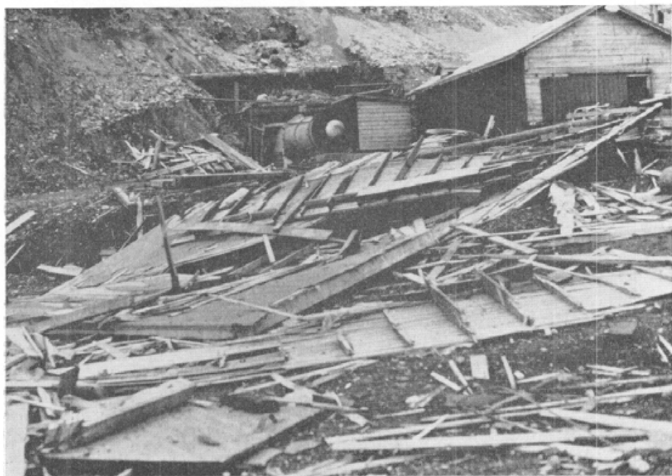
Plate XB. Balmer North mine. Portal of No. 2 or intake tunnel showing wreckage of fan-house. Fan was moved from left of portal to present position to re-establish ventilation.
