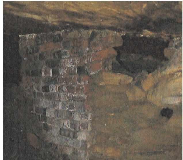
Photo 2. Original firewall of brick and stone, on north side of underground ventilation furnace, inby Portal 5. Sandstone roof above furnace has been baked and reddened, and shows minor flaking.
