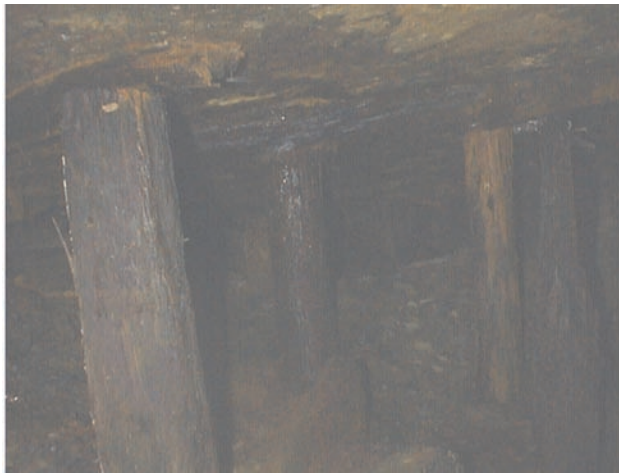
Photo 1. View southward into workings inby Portal 4. Timber posts are 20 to 30 cm in diameter, and have single cap-pieces to spread load against carbonaceous mudstone roof of coal bed.
