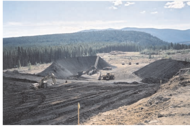
Photo 3. Basin Coal mine near Coalmont. The stripped but unmined coal seam is in the foreground with screened, raw coal on the pile near the conveyor. Photo courtesy of Eric Beresford, Compliance Energy Corp.
