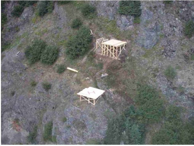
Photo 10. Drill platform under construction at the Rico gold vein showing on the Kalum property.
