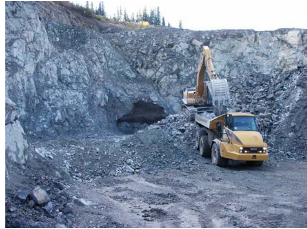
Figure 3-5. Stripping waste rock from the Creek zone open cut, Shasta gold-silver mine.
