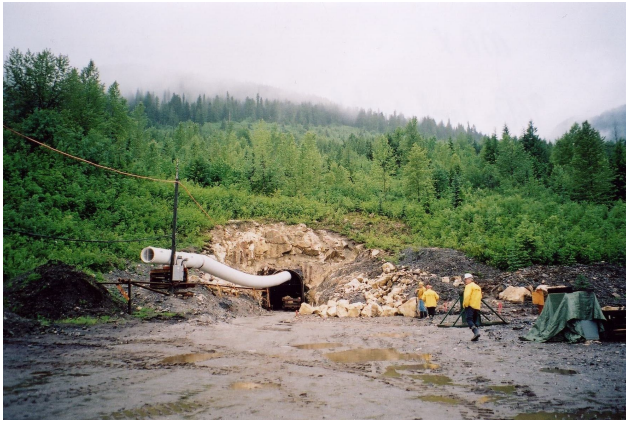
Photo 8. Portal area at the MAX molybdenum site being readied for production in late 2006.
