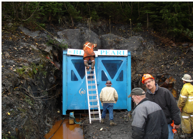
Figure 2.17. Erecting the sign above the new doors at the 1066-level portal, Davidson molybdenum deposit.
