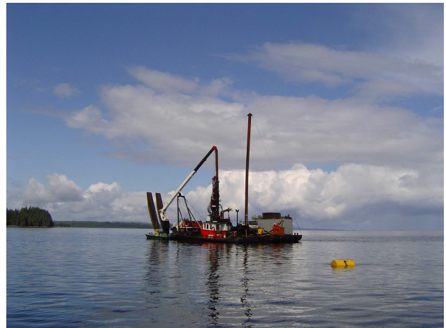
Figure 6.9. Marine drill rig for geotechnical testing of the ship loading facility site of the newly certified and permitted Orca Sand and Gravel project near Port McNeill.
