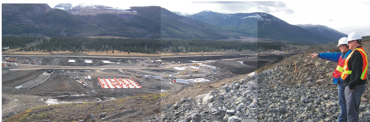
Figure 7.5. Western Canadian Coal Corp Vice-President/COO John Hogg and Senior Mine Engineer Gary Gould looking southward over construction taking place on the Wolverine mine-site.
