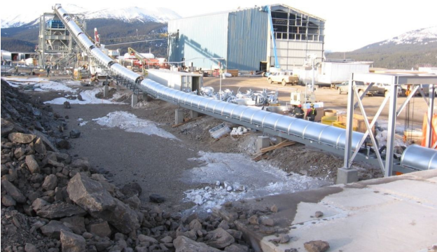
Figure 7.4. Coal processing plant under construction at the Trend Small Mine (photograph courtesy of Kevin Sharman, NEMI).
