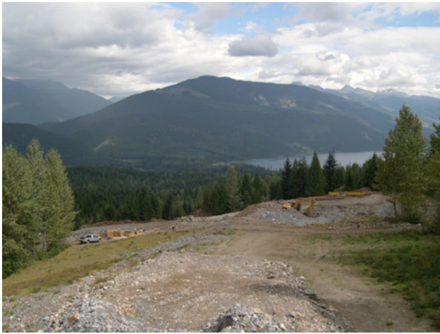
Photo 5. Looking northeasterly over the millsite construction area towards Trout Lake, MAX project (photo by T. Schroeter).
