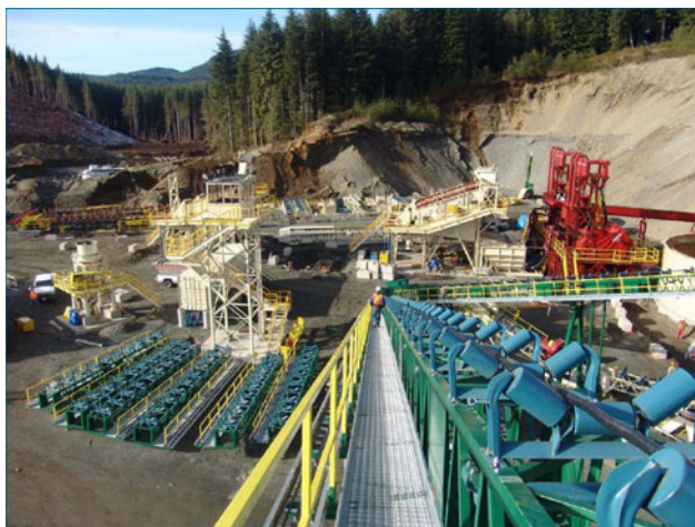
Photo 4. Orca sand and gravel operation near Port McNeil, northern Vancouver Island. Preparation of new conveyor belt system.
