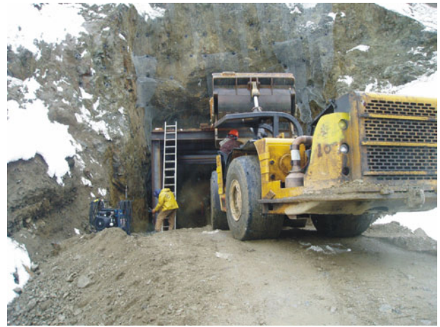
Figure 4.14. Development of the North zone portal, QR gold mine (photograph courtesy of Jim Miller-Tait).
