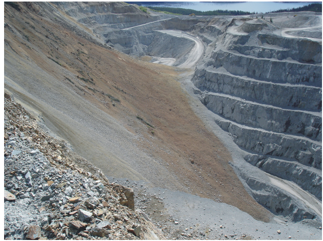
Figure 1.4. Wall failure ended mining in the East pit at Huckleberry mine.
