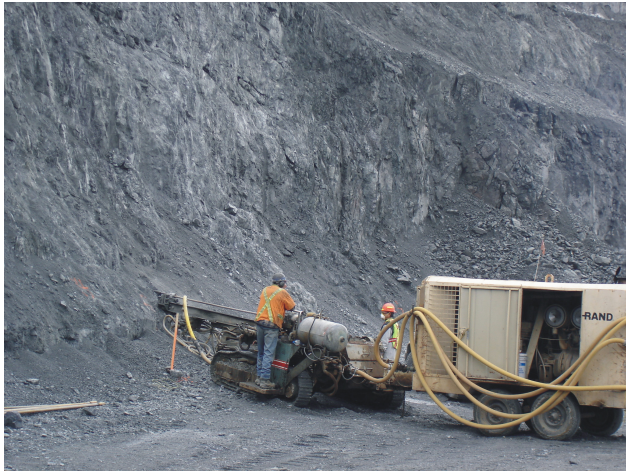
Figure 1.5. Drain holes are drilled in the highwall of the Main Zone Extension pit at Huckleberry mine.
