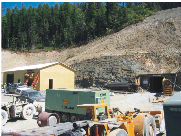
Figure 6.5. The Lexington portal and surface facilities on the Greenwood Gold Project, Merit Mining Corp.
