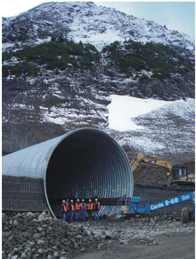
Figure 1.8. North portal of the Galore Creek access tunnel, entrance to the mine site in development.
