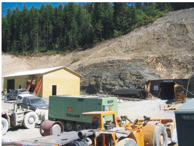
Figure 6.5. The Lexington portal and surface facilities on the Greenwood Gold Project, Merit Mining Corp.
