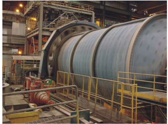
Figure 3.8. Ball mill in operation in the Kemess mine concentrator.
