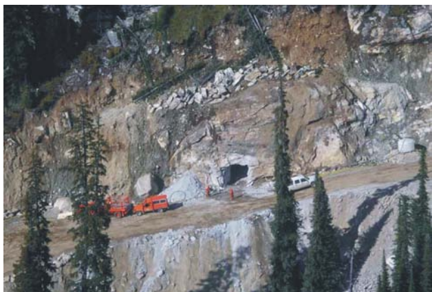
Figure 4.13. Portal to permit year round drilling of the E-Zone and Creek Zone at the Ruddock Creek property of Selkirk Metals Corp (Photo courtesy of Selkirk Metals Corp).
