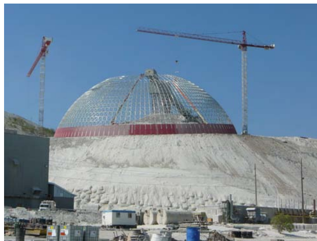
Figure 4.5. Geodesic domes over ore stockpiles being installed at the Highland Valley Copper mine near Logan Lake.
