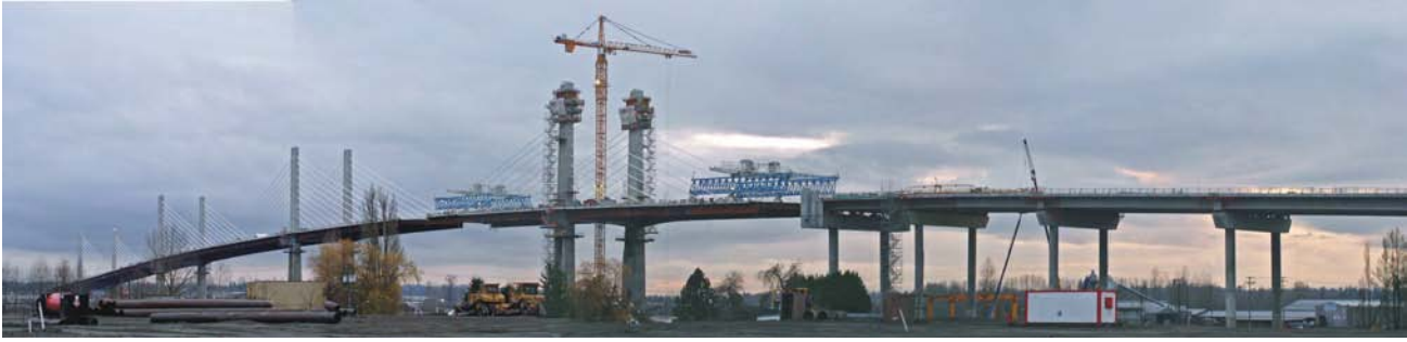
Figure 5.7. Golden Ears Bridge construction, Lower Mainland, as of early December 2008. In addition to fill, infrastructure projects such as this typically require high quality aggregate and other construction materials that can meet specific engineering standards.
