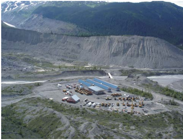
Figure 1.9. Galore Creek, construction camp and equipment at Km 89.5, a stranded segment of the access road to the copper-gold deposit.
