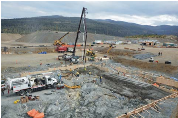
Figure 4.12. Foundations being poured this fall will allow the construction of a new mill building at the Copper Mountain mine development to begin in the spring of 2010 (photo courtesy of Copper Mountain Mining Corporation).
