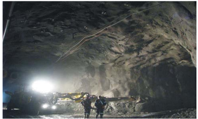
Figure 4.9. A Jumbo at the New Afton mine development site which now includes over 5 km of underground development and a 4.5 km conveyor decline that is nearing completion (photo courtesy of New Gold Inc).
