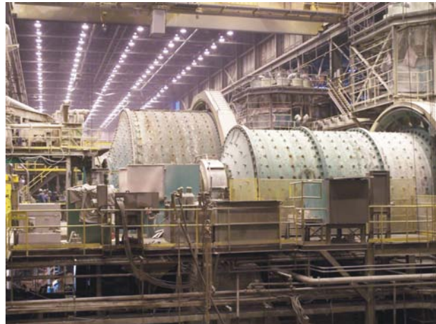
Figure 4.6. The mill at the Highland Valley Copper mine which processed approximately 44 Mt of ore in 2009.
