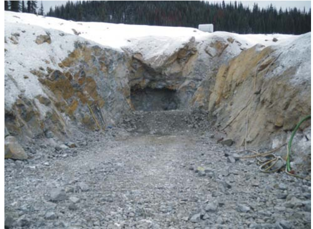
Figure 4.16. The start of a portal to exploit the Jewelry Box vein at the Bonaparte Gold property of Encore Renaissance Resources Corp north of Kamloops.
