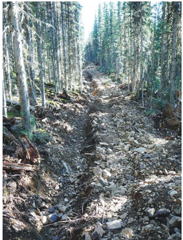
Figure 4.17. One of many lengthy trenches at Molycor Gold Corp's Windpass property near Little Fort.
