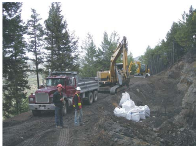
Figure 4.18c. At the Watson Bar property. Loading the bulk sample into a haul truck in preparation for direct shipping to the custom mill.
