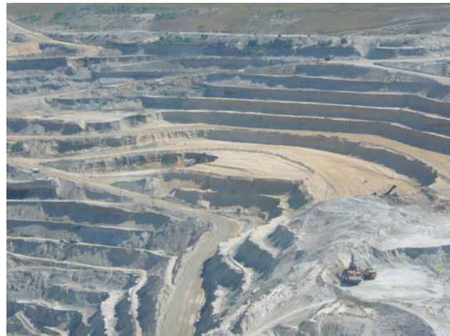
Figure 4.5. Overburden stripping at the east wall expansion of the Valley pit at the Highland Valley Copper mine near Logan Lake.
