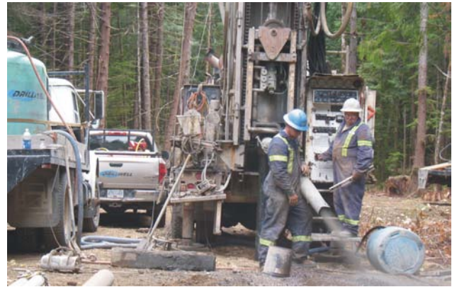
Figure 5.18. Driving in casing for a drill hole on the Raven coal project.
