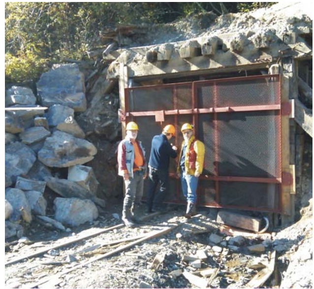
Figure 5.17. The portal at the former Carolin Mine was re-timbered as part of the underground rehabilitation at the Ladner project. Photo courtesy Module Resources Incorporated.
