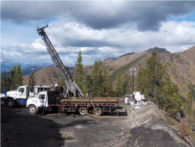
Figure 6.9. View looking north of rotary drilling at the north end of Teck Coal Limited's Mount Michael property.
