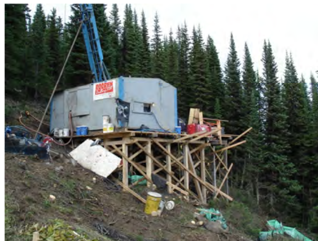
Figure 27. Akie, large drill platform to support a drill rig for deep holes.
