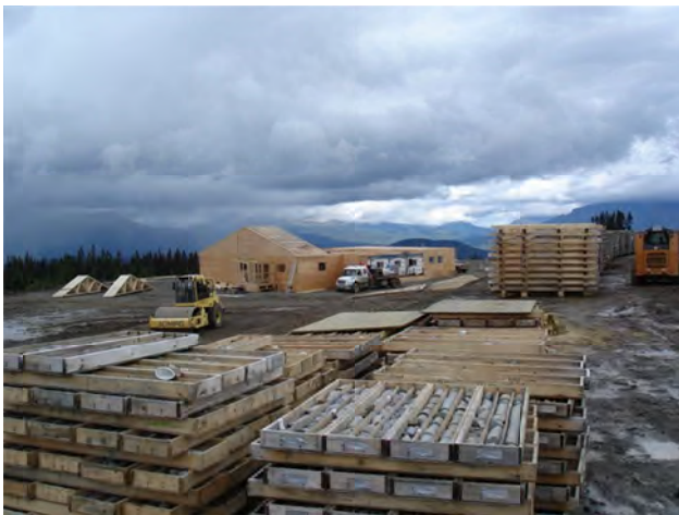
Figure 16. Red Chris copper-gold project; new core shack under construction, the old core shack is in the area of proposed pit development.
