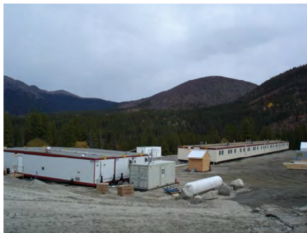
Figure 67. Silvertip; a new 49-man camp was installed on the silver manto prospect that is suitable for exploration and, in the future, a mining crew.
