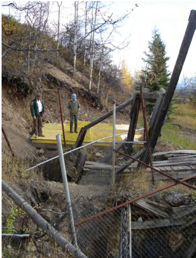
Figure 58. Silver Queen project; covers were installed on historic underground workings for safety reasons.
