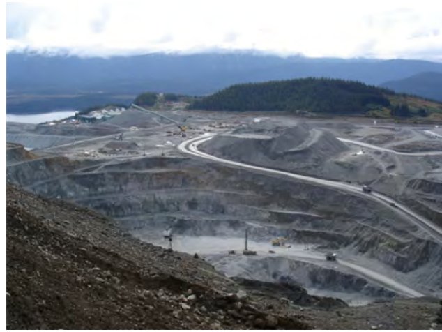
Figure 6. Huckleberry copper mine; mining in the MZX pit in September 2010, low grade stockpile and mill in the background.
