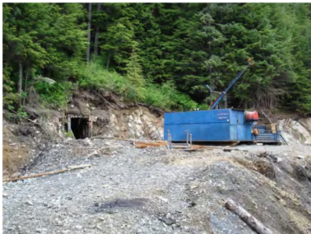
Figure 80. Dunwell project; drill set up at the portal of the past-producing silver-gold mine.
