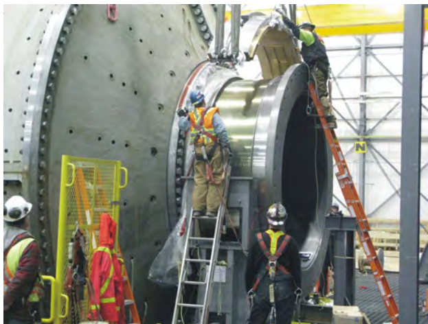
Figure 11c. Fitting a bearing on a mill (photo courtesy of Copper Mountain Mining Corporation).
