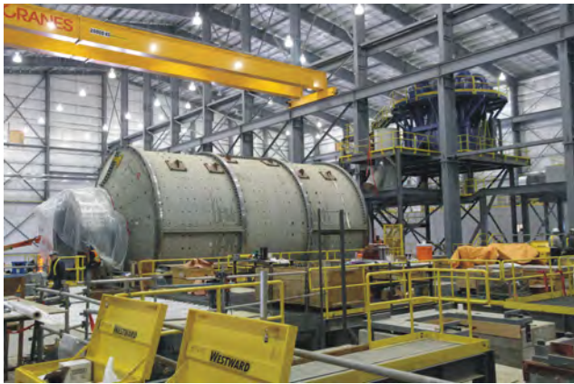
Figure 11b. By the fall of the year major mill components were installed at Copper Mountain (photo courtesy of Copper Mountain Mining Corporation).
