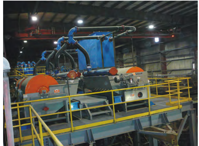
Figure 8. A newly installed magnetite recovery circuit at the Mount Polley mine will provide magnetite for a variety of uses, including the cleaning of coal.
