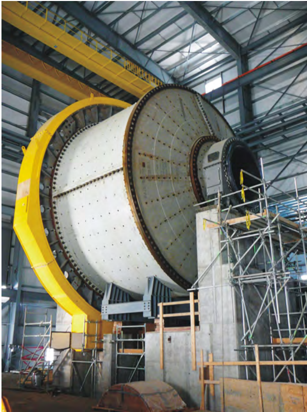
Figure 9. A partially installed 28 foot SAG mill at the New Afton gold-copper project near Kamloops awaits a mid-2012 start-up.
