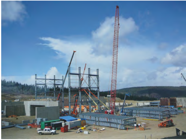
Figure 11a. Flying steel for the new mill building at the Copper Mountain copper-gold project near Princeton started in April 2010.
