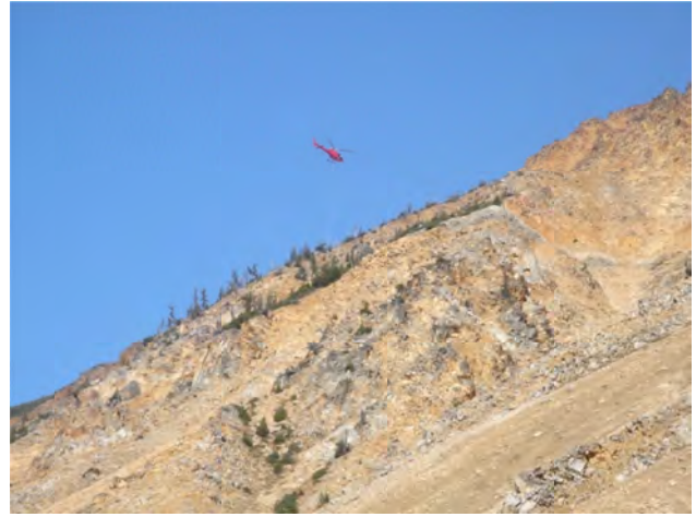
Figure 22. A helicopter slings a rig in for a setup on Float Creek at the Salal Creek project. Photo courtesy Miocene Metals Limited.
