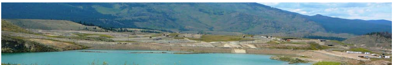
Figure 7. Site work is well underway at the New Afton project where a new tailings storage facility is being constructed and the Afton pit is being dewatered into the former Pothook pit.
