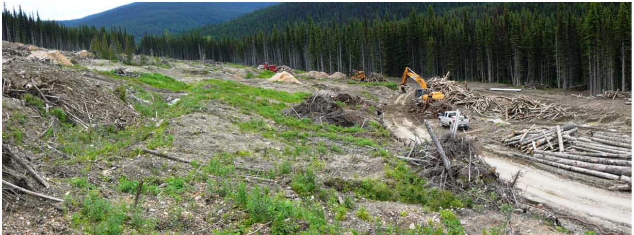
Figure 5. Site preparation is underway on Barkerville Mountain where the new Bonanza Ledge mine has been permitted
