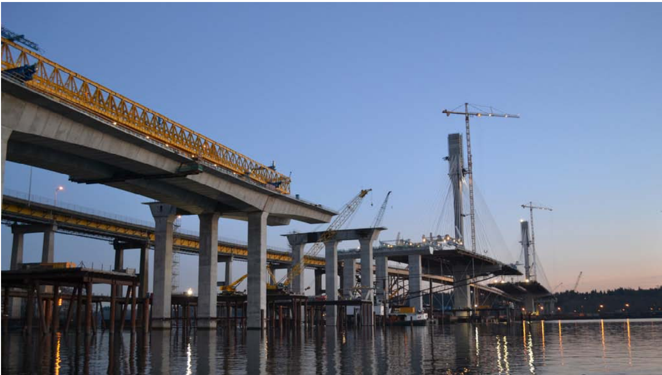
Figure 10. Supporting demand: infrastructure projects such as the Port Mann project, part of the Gateway Program established in 2003, contribute substantially to demand for aggregates in the Lower Mainland market.
