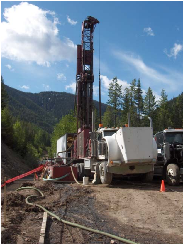
Figure 18. Rotary drilling on the Coal Creek Project (Crowsnest Pass Coal Mining Ltd).
