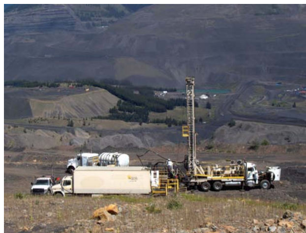
Figure 15. Rotary drilling on the Swift Project, Fording River Operations (Teck Coal Limited).
