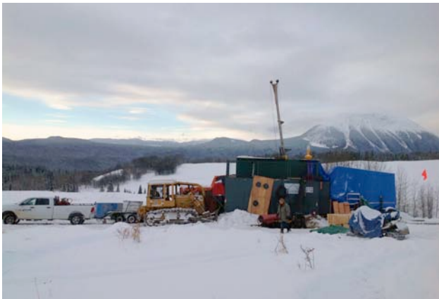
Figure 2.26. Exploration drilling at the Itsit porphyry prospect resumed in late November. Due to overlapping land use interests, all drilling fluids are required to be contained and disposed of in the historic tailings impoundment area at the nearby Silver Queen mine.
