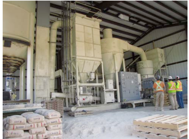
Figure 2.6. Mine Inspectors Doug Flynn and Rebecca Misener take a closer look at the former flour bagging plant now re-fitted and reinforced for barite at the Fireside mine site
