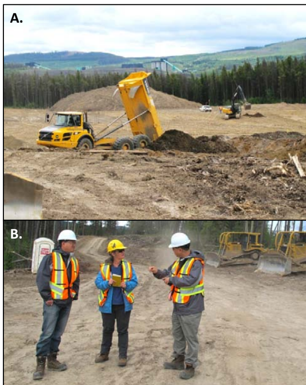
Figure 3.11. Murray River – A. Stripped and graded North Shaft site with soil stockpile and Quintette Mine in the background 3 km to the southeast; B. HD Mining Engineers discuss North Shaft site with Janet Riddell.
