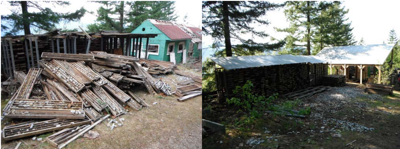
Figure 5.15. Before and after repair shots of the core storage and logging area at the Abo gold project. Vandalism and theft are intractable problems at accessible locations. This core was apparently dumped to gain access to the rebar used in the racks.
