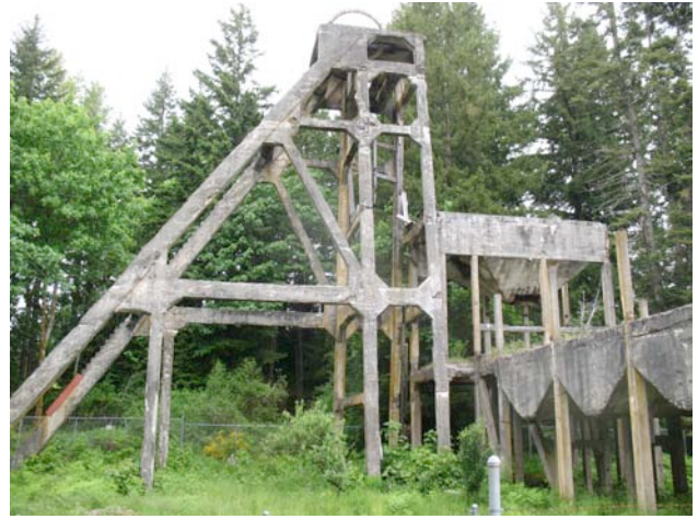
Figure 5.6. The concrete headframe of the Morden Mine, built in 1913. Though it was not a particularly successful operation (it closed in bankruptcy in 1921), it stands as a reminder of a previous era of coal mining on Vancouver Island which began in 1849. Vancouver Island's coal resources are far from exhausted. The Morden Mine itself may have as much as 7 million tonnes resources (but is located in a park in a rural/residential setting).
