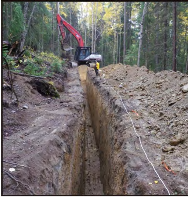
Figure 22. Green Gold – Trenching to bedrock in the Pinchi Fault zone, 36 km southwest of Prince George.
