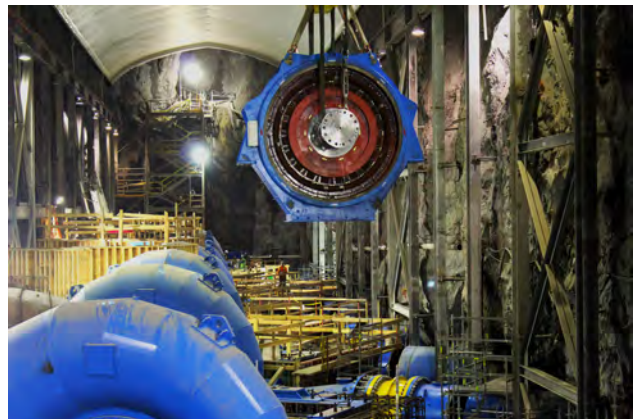
Figure 12. Turbine installation at Alta Gas's Forrest Kerr run-of-river 195 MW hydroelectric power plant which will feed into the Northwest Transmission Line. Photo credit Lorne Kelly, Alta Gas.
