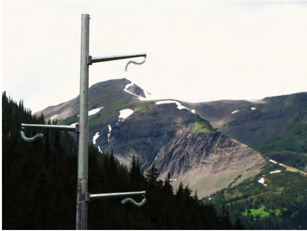
Figure 3. Newly constructed Northwest transmission line tower with recently hung insulators with folded Bowser Lake Group sediments in the background.
