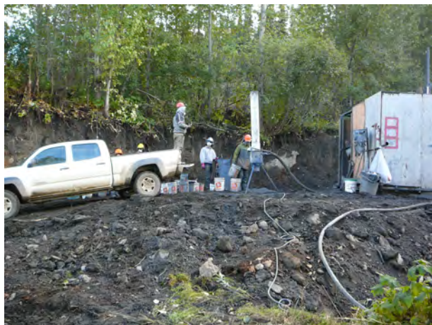
Figure 7. Preparing to collect samples from reverse circulation drilling at Spanish Mountain gold-silver project. (Jim Britton photo)
