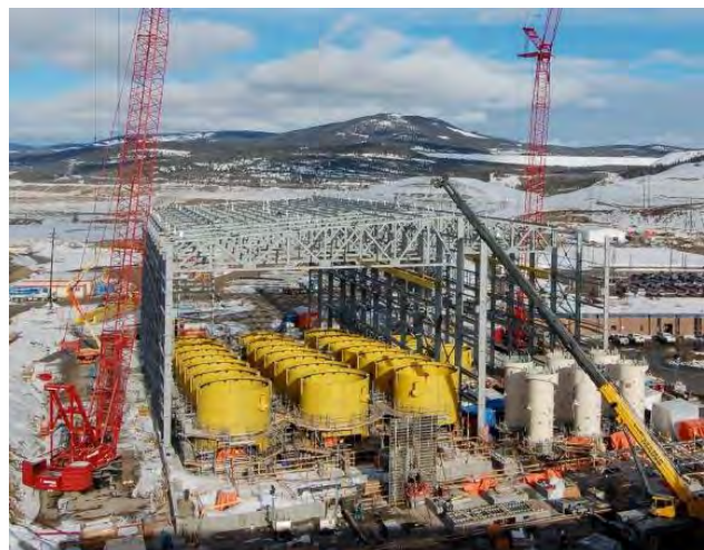
Figure 5. New mill under construction at Highland Valley Copper mine. (Image courtesy of Teck Highland Valley Copper Partnership)
