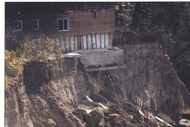
This structure near Williams Lake received considerable damage in 1992 from undercutting of the slope (photo courtesy of the Ministry of Health).
