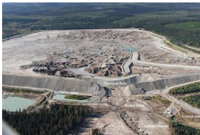
Fig. 6. Repairing the breached tailings dam at Mount Polley mine, September 2014. Photo courtesy of Imperial Metals Corporation.
