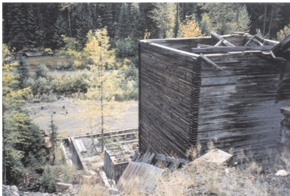
Photo 53. Unknown mill near Sandon, B.C. The mill could not be linked to specific mine sites.
