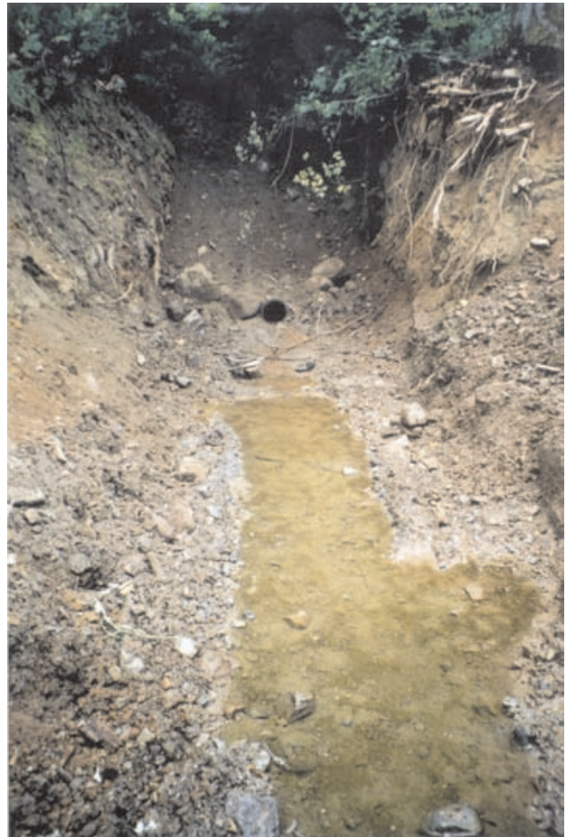
Photo 56. Unknown backfilled adit (UTM coordinates: 0441519, 5437741) on Monte Cristo Mountain., Rossland, B.C.
