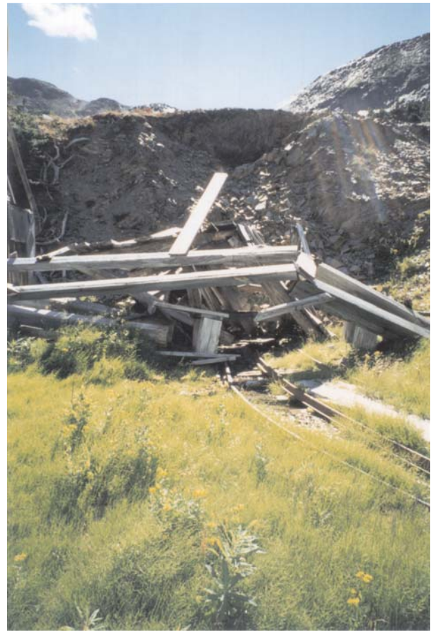
Photo 4. Native (Lorraine) caved portal and waste rock dumps. Drainage flows from the adit.
