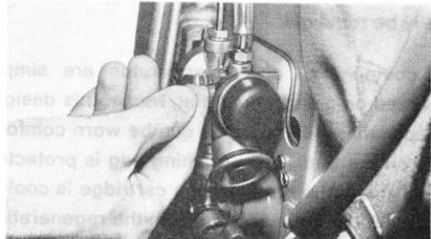
Fig. 9 Closing the shut-off valve
