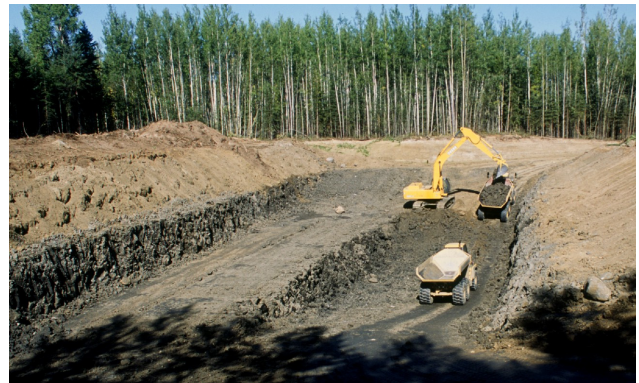
Figure 4. Excavation of till from a borrow pit for construction of a well site access road. Photo R. Smith.
