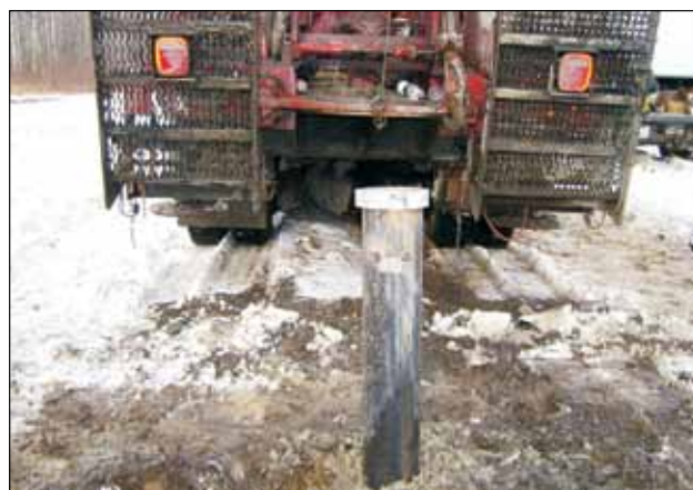
Figure 6. Following completion, approximately 1.5 m of steel casing remained above ground to mark the well. The casing was tagged with a well number and a lock cap was installed.
