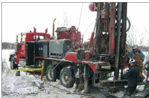
Figure 5. In November 2011, six new water observation wells were drilled along on road rights-of-way using an air rotary water well drilling rig with a casing hammer.
