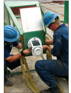
U.S. Coast Guard personnel retrofitting a buoy tower with Carmanah Model 702 light
