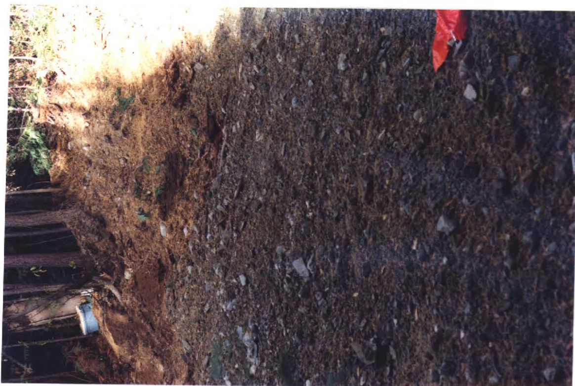
Photo 27- The upper old prospector holes were sampled and then filled in with the Excavator and smoothed over. This was the start of the Reclamation of the Mine site.
