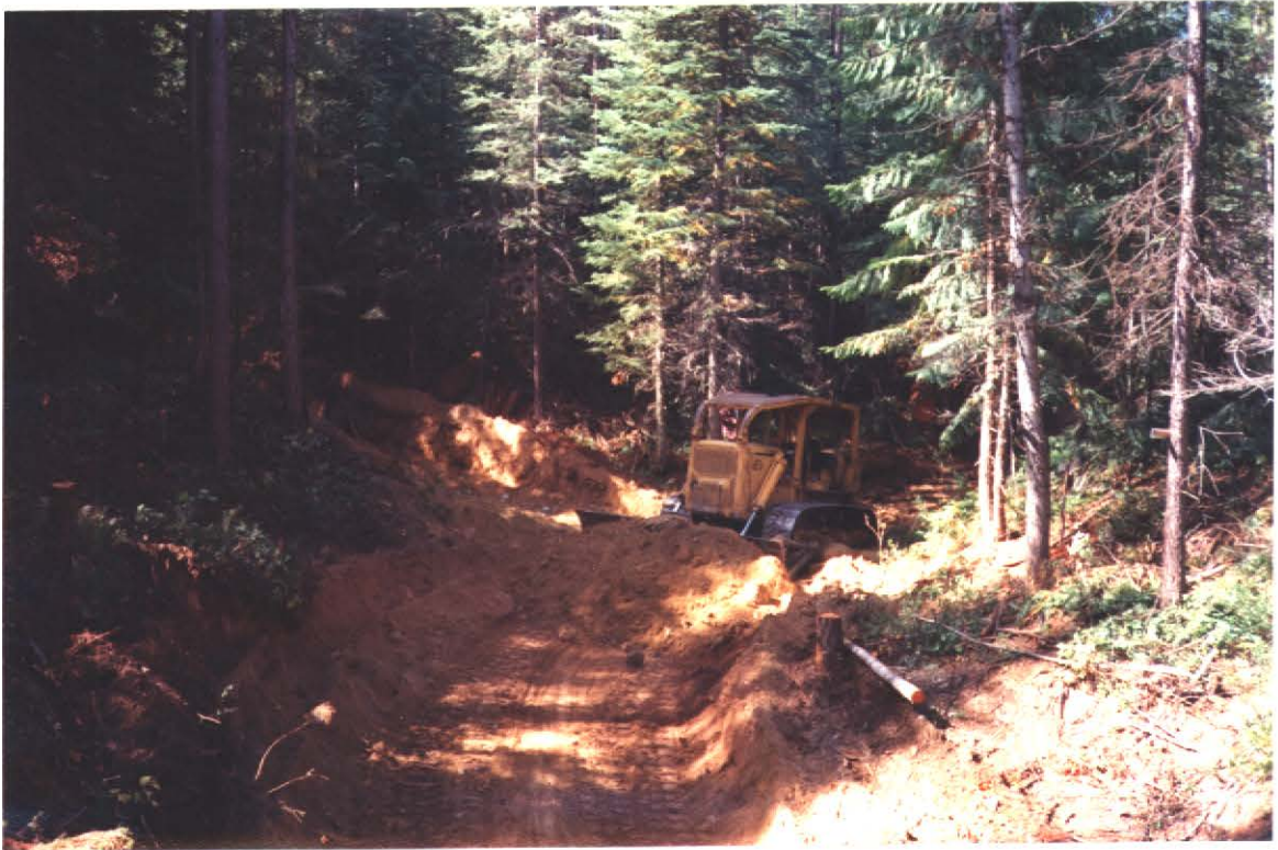
Photo 8- After hand clearing and piling brush a D-7 Cat was brought in to improve trails and improve the primary gullie to be excavated
