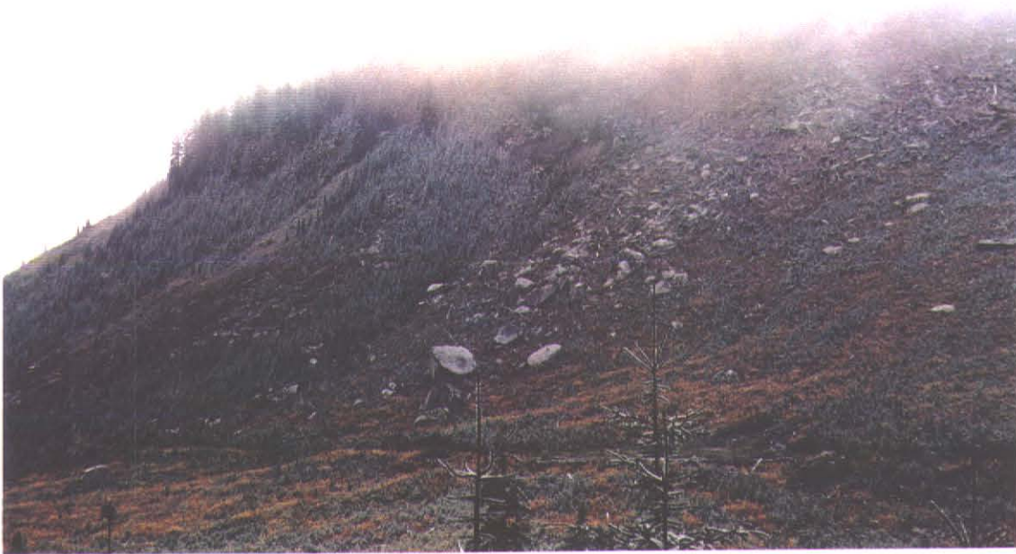
Photo 4.3 - Large boulders above road at location 4.3.
