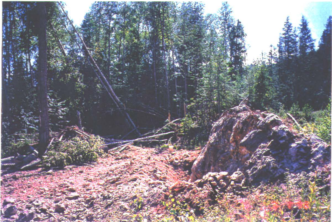
Trench #1 - Photo #6 Foreground is Trench #1. In the background is Trench #2 after the blast
