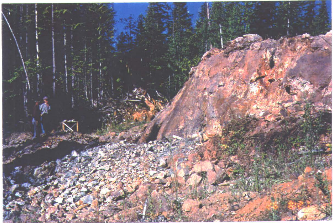
Trench #1 - Photo #3 Same picture as photo #2 above, view in opposite direction. Dave & Camille standing in front of showing prior to blast for Trench #2. Trench #1 in the background
