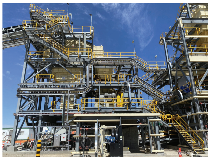
Fig. 6. Blackwater's gold mine crusher (Artemis Gold Inc.).
