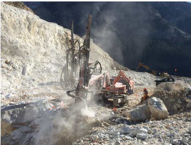
Fig. 14. Blast hole drilling at the Mount Brussilof mine, which produces magnesite from Cambrian carbonates of the Cathedral formation.
